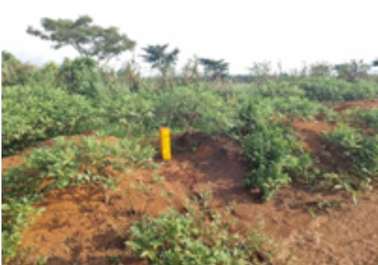
A few months after the topsoil was put back, Lantana camara has partially invaded the ROW
